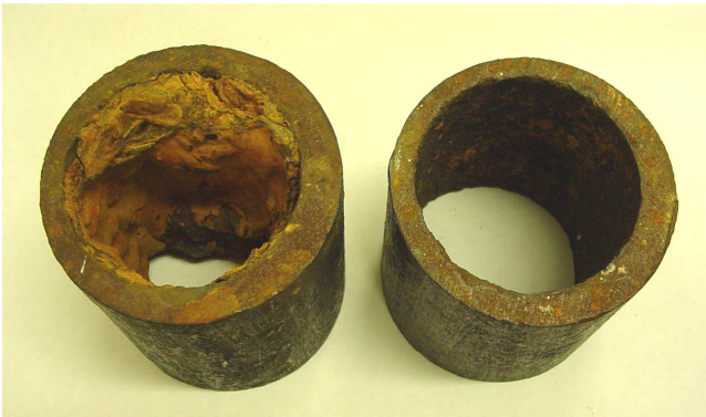
Fig. 9. Example of effective cleaning of a water pipeline after 50 years of use
